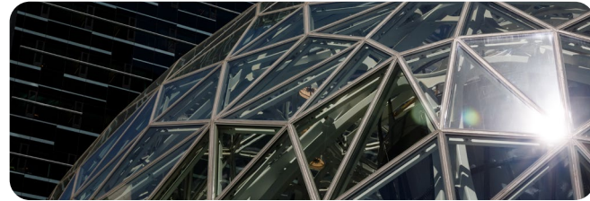
The thousands of panes of glass in The Spheres are designed to maximize light exposure for plants while maintaining a consistent temperature inside.
